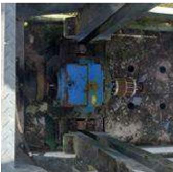
Figure D Corroded Motor
