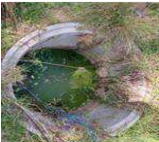
Figure A Overgrown Manhole
