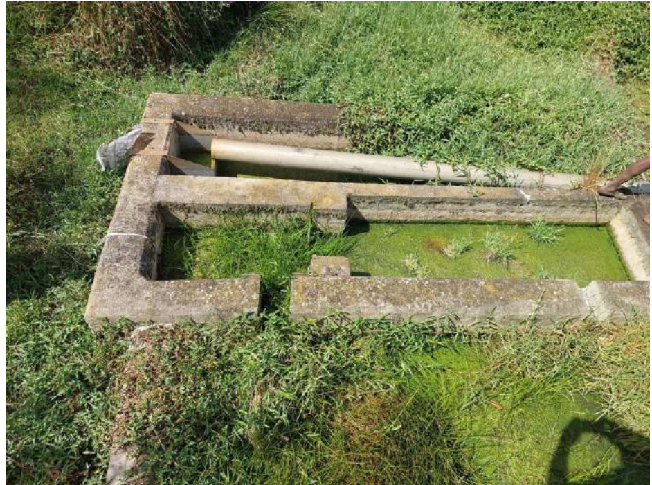
Figure C Overgrown Sedimentation Tank
