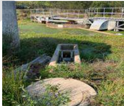
Figure H Overgrown Sedimentation Tank
