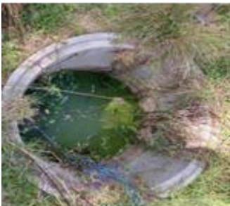
Figure A Overgrown Manhole
