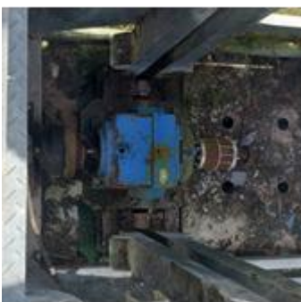
Figure D Corroded Motor
