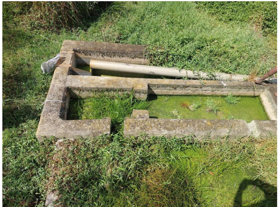
Figure C Overgrown Sedimentation Tank
