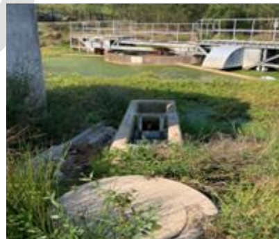
Figure H Overgrown Sedimentation Tank
